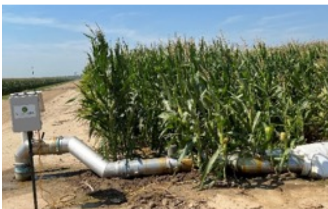
Figure 1. Actuated valve in a corn field.
